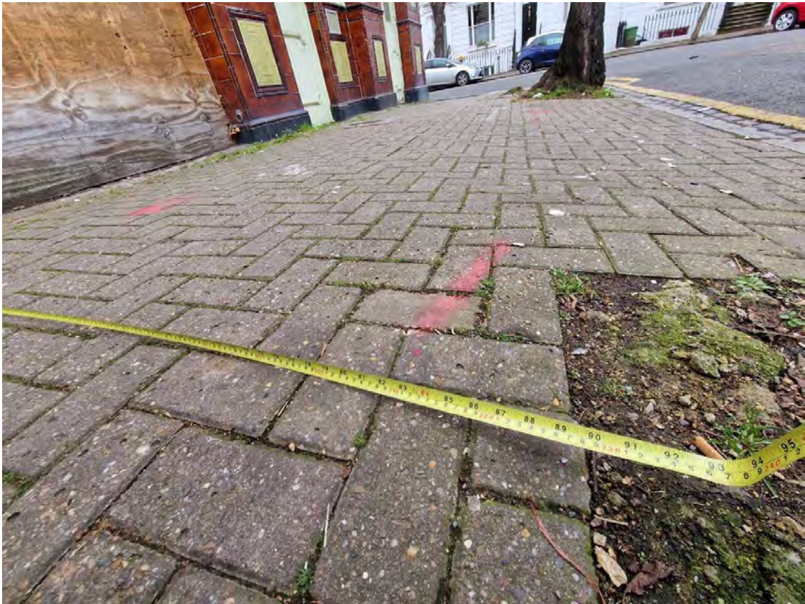
Pavement on East side of 50 Florence Street is just under 2.3 metres wide.
